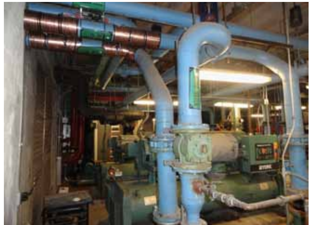
Vulcan S100 units installed on the double chiller
