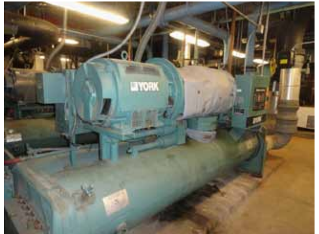
Vulcan units protecting chiller pumps from scale and rust
