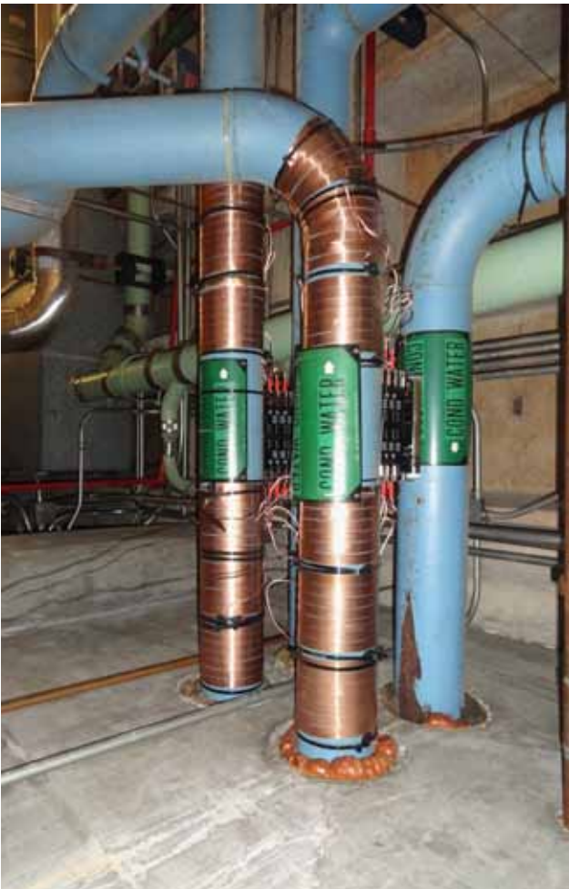
Vulcan S100 units installed on the double chiller
