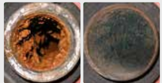
Biofilm in a piping system
