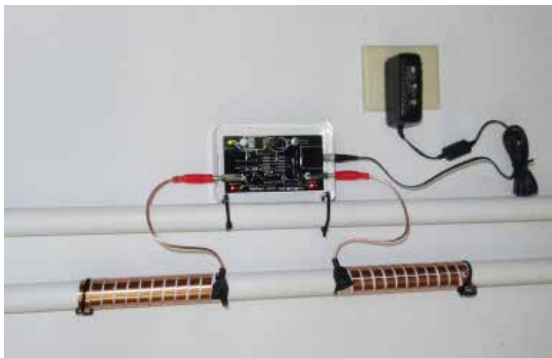
Picture 4: General arrangement of the physical water treatment
